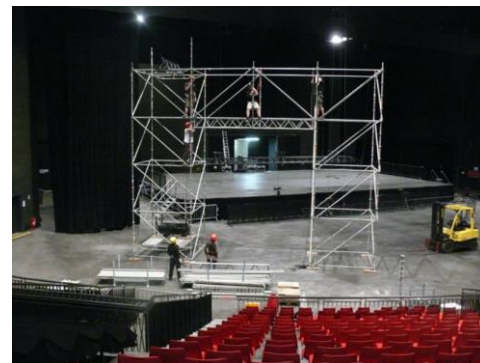
Techniciens structure @ Prolive formation
